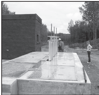
Mole Lake’s new wastewater treatment system.
